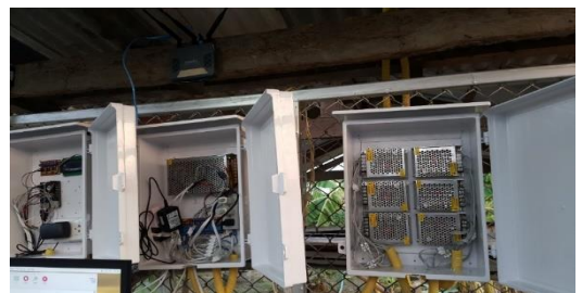
Figure 14. Water pump and NPK fertility pump control set
