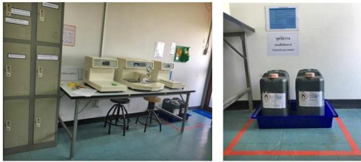
Figure 8. The appropriate waste container specifically for flammable chemical and stored away from heat, fire sources and flame (after the implementation)
